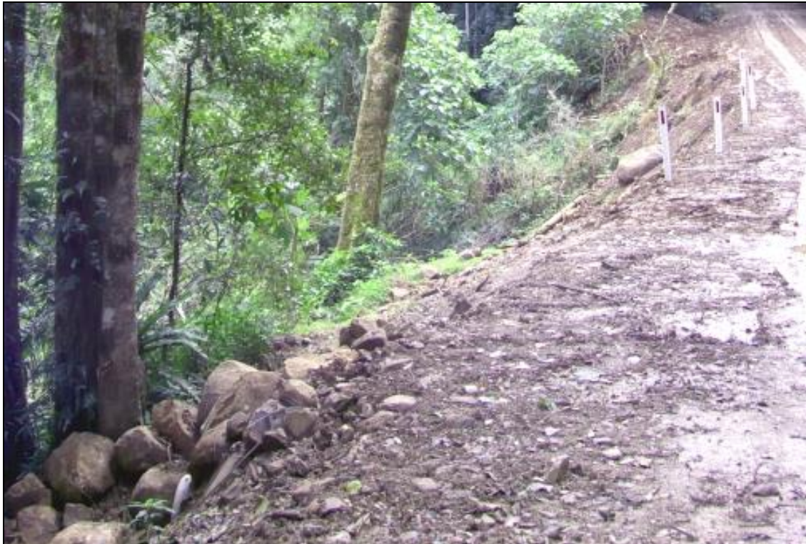
Figure 5. Sheet erosion and roadside slumping.
